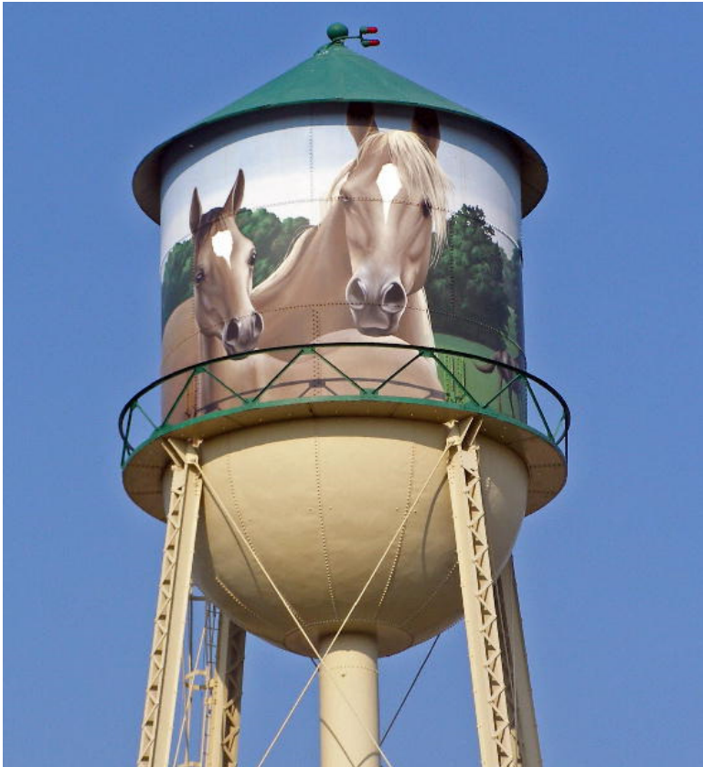
Photo of the water tower at the Equestrian Center in Upper Marlboro, Maryland. Courtesy of www.radiojeep.ceureka.com
