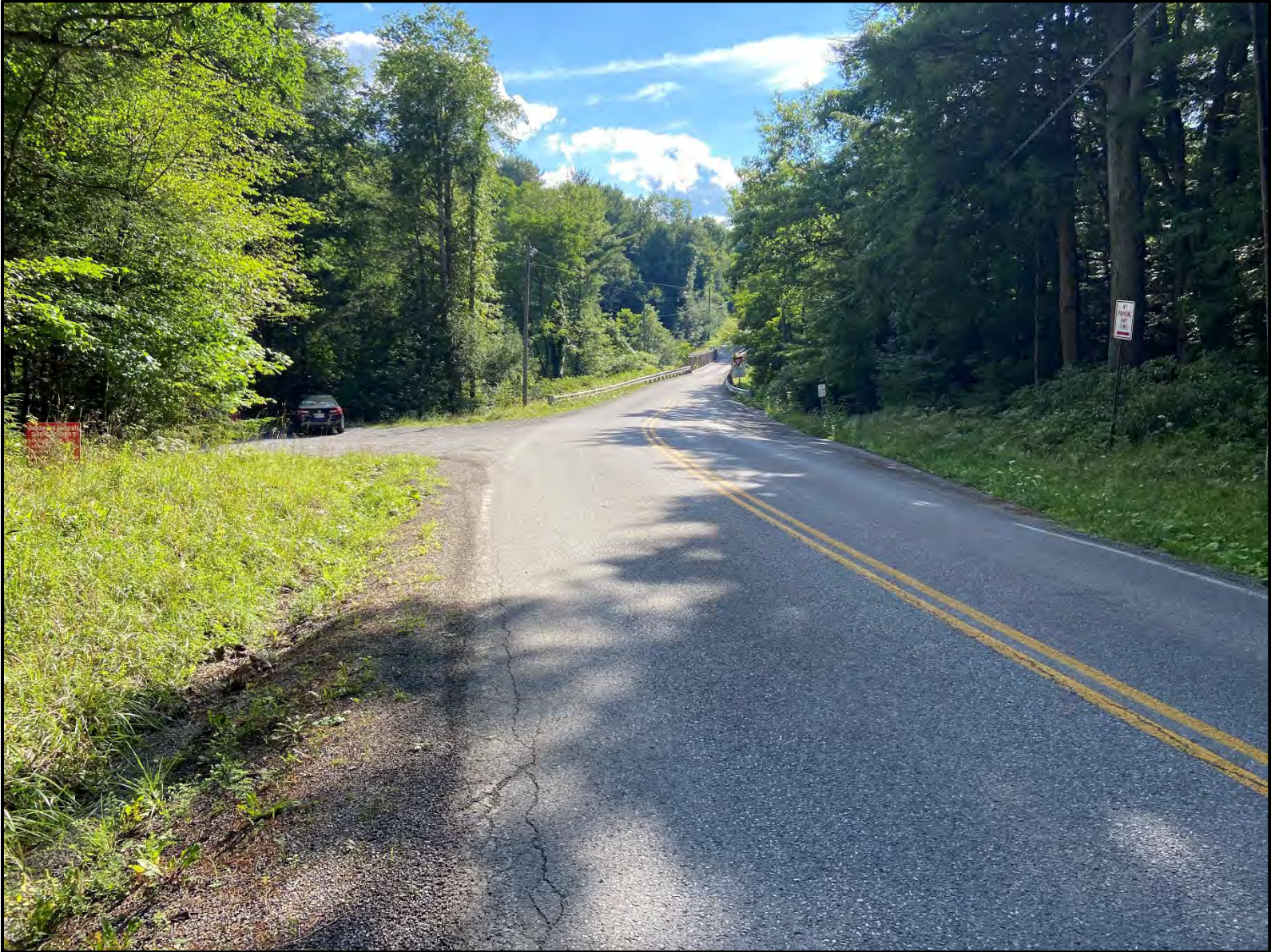
Existing Conditions of the eastern approach to the Swallow Falls Road Bridge.
