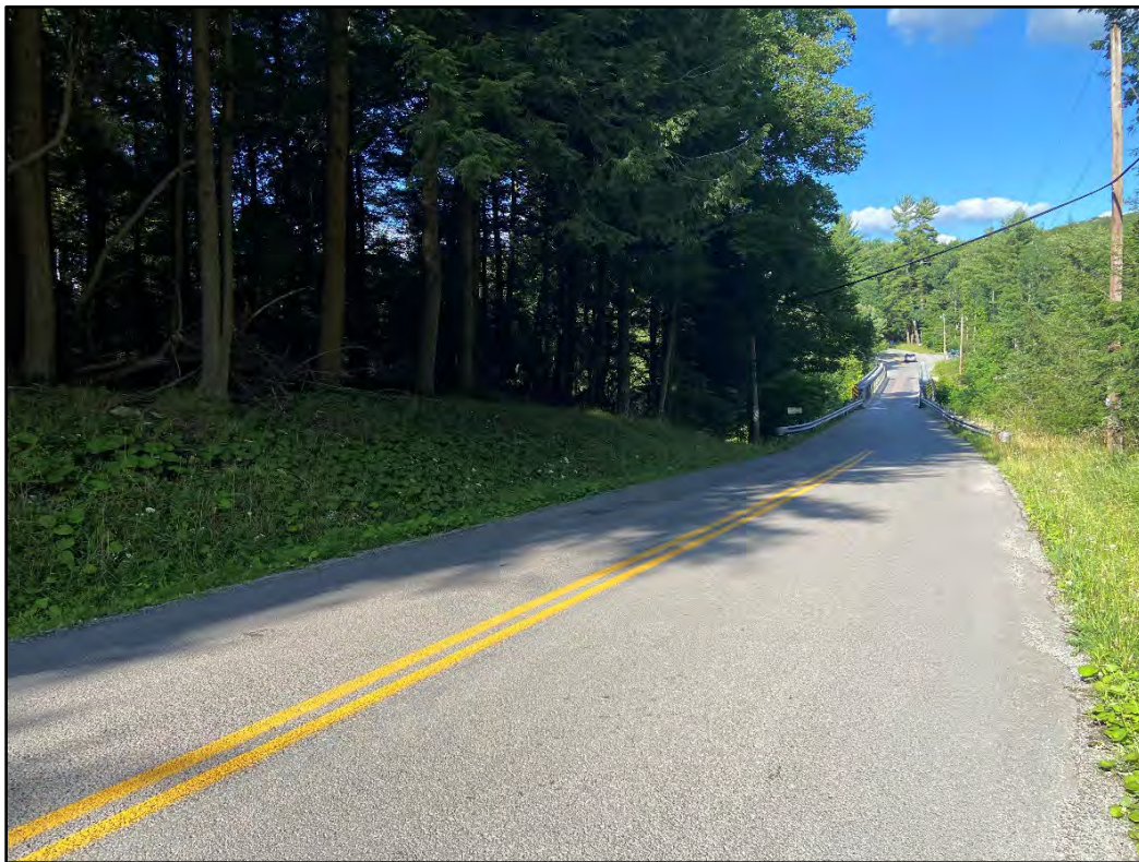
Image 8 - View of the bridge approach on Swallow Falls Road, west of the bridge.
