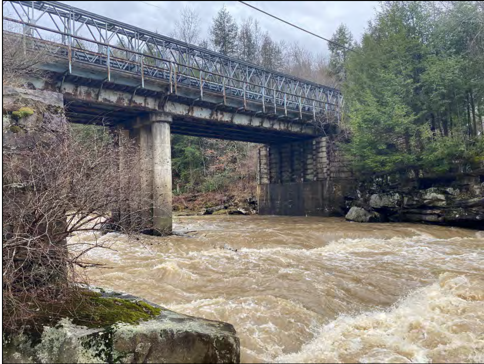
Image 9 – View of the Swallow Falls Road Bridge from the eastern bank of Youghiogheny River, north of Swallow Falls Road. Visible are the abandoned stone abutment (left), the existing in-river center pier, and concrete abutment of the bridge (right).
